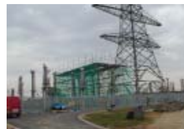
Sealing end compound.
